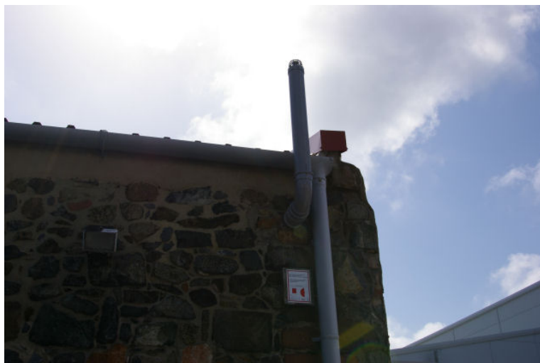
Figure 5 - Antenna at PoP is disguised as a gutter downpipe
