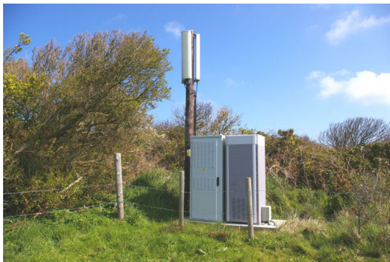
Figure 7- Antennas at Little Sark are high power and are only ~4m high
